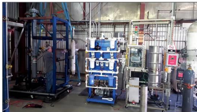
Intellergy's Engineering GTL Plant at UC Berkeley
